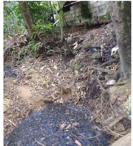
Wastewater leaks from an eroding piggery in the Achugao watershed. This piggery owner moved the pigs to a new location away from the stream.
