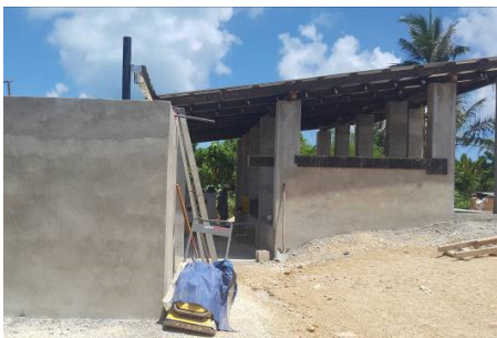
The finished piggery includes a waste storage facility, roofs and covers, roof runoff capture structure, and heavy use area protection.
