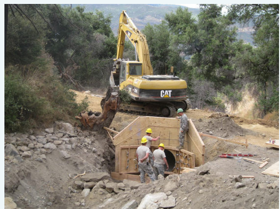
The Tribe received technical assistance from the U.S. Department of Defense's Innovative Readiness Training Program , which provides training and readiness for military personnel while addressing the needs of underserved communities. The personnel helped fix road and culvert damage from the 2007 fires.
