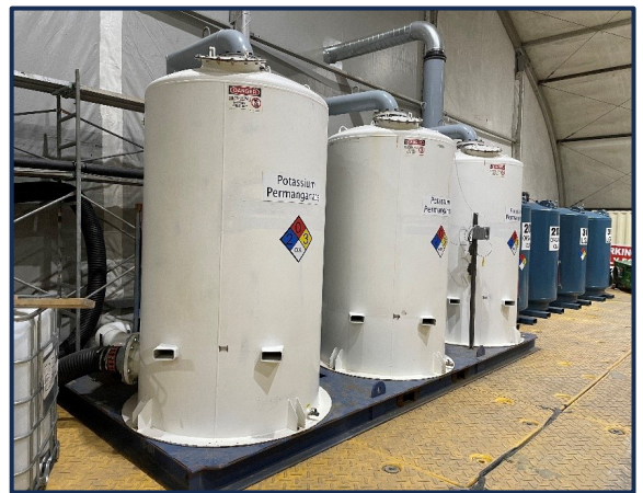
Photo 3 shows a treatment area within the on-site wastewater treatment plant.
