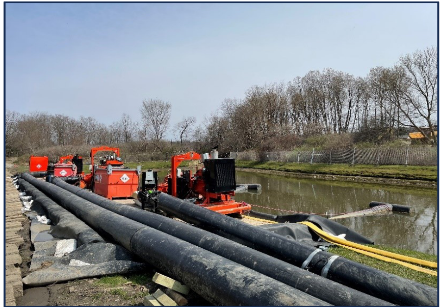
Photo 1 shows the current bypass system which carries water to Sulphur Run.
