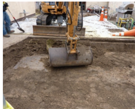
Colorado Smelter cleanup crews excavate contaminated soil from a residential property in Pueblo, Colorado
