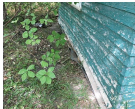
Brownfields Cleanup, Spirit Lake Reservation. Photo of an abandoned building contaminated with asbestos, lead-based paint, and lead in the soil.
