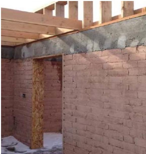
The Apsaalooke Crow Tribe used Crow resources and tribal member labor to build compressed earth block homes. Photo: Apsaalooke Housing Authority
