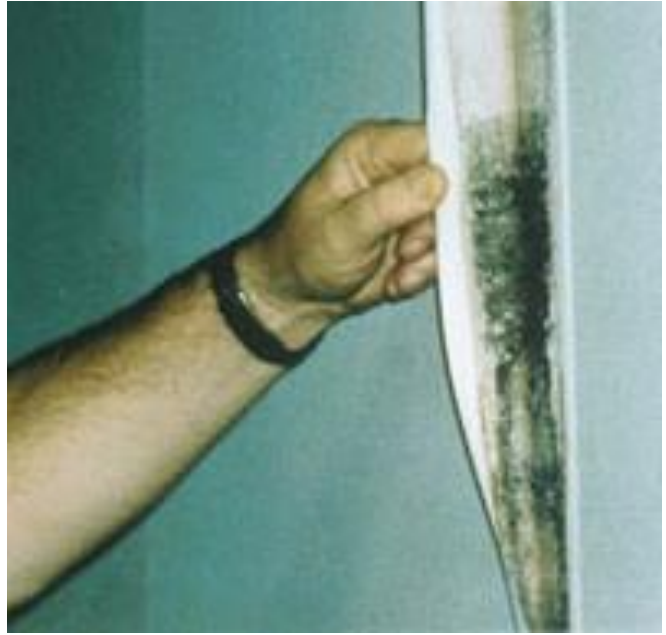
Hidden mold growing behind wallpaper.
