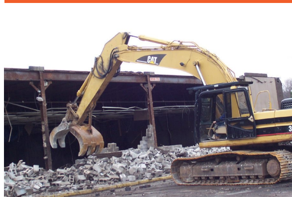
During the demolition and debris removal phase of the project (photo credit: Paul Testa).
