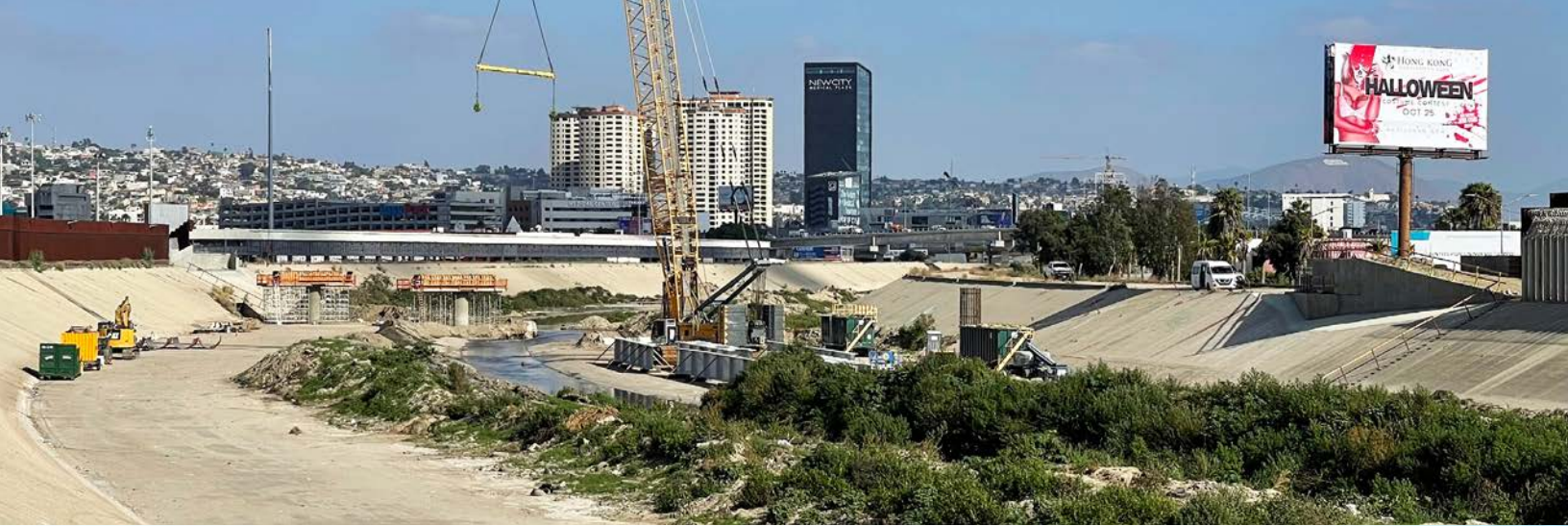
Construction of border wall with hoistable gates across the Tijuana River channel in San Diego in 2023, as described on page 33. Photo credit: Paul Ganster
