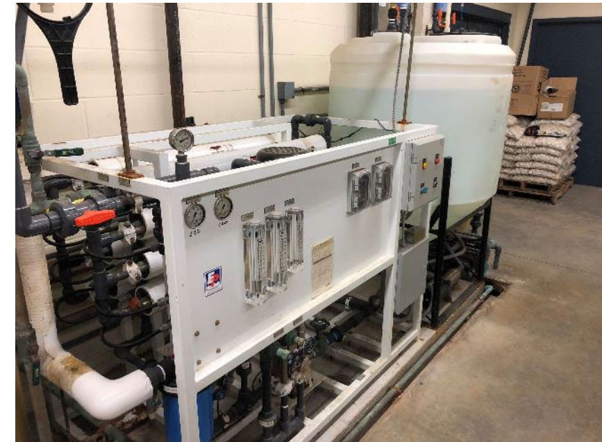
Lab RO treatment system
