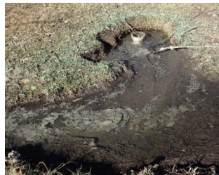
Sewage flowing from a sewer cleanout pipe and into a ditch
