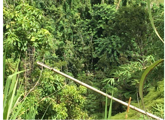
Aboveground drinking water distribution pipe in rural Puerto Rico broken as a result of a hurricane. (EPA OIG Photo)
