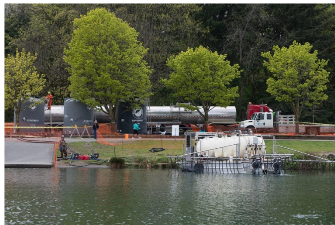
Three on-shore alum storage tanks are being filled from tanker trucks in the background. On the water, there is a barge with alum distribution tanks and lines.
