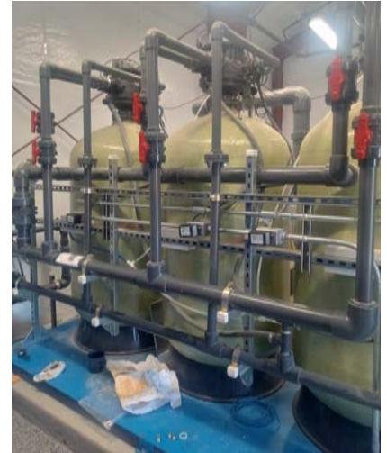
New filtration equipment installed at the Big Valley Rancheria drinking water treatment plant.
