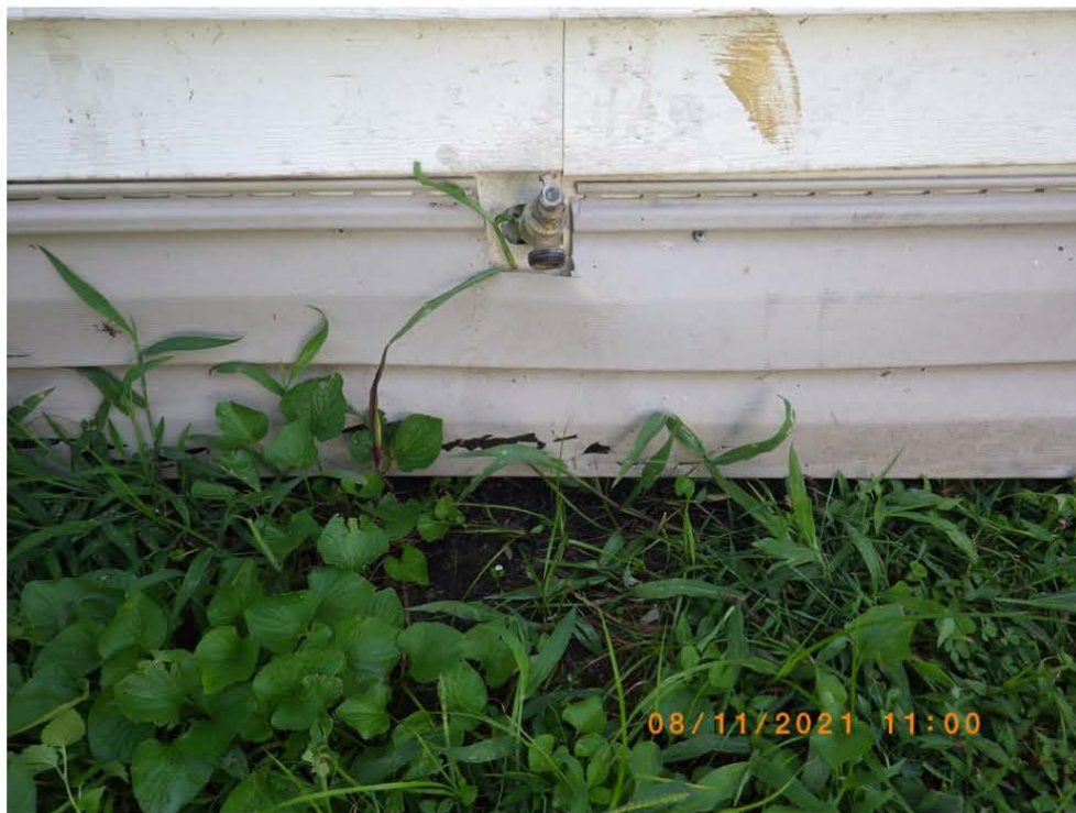
RIMG1467 Hose bib at site 1-05, 5949 Piat Pl, 8/11/21
