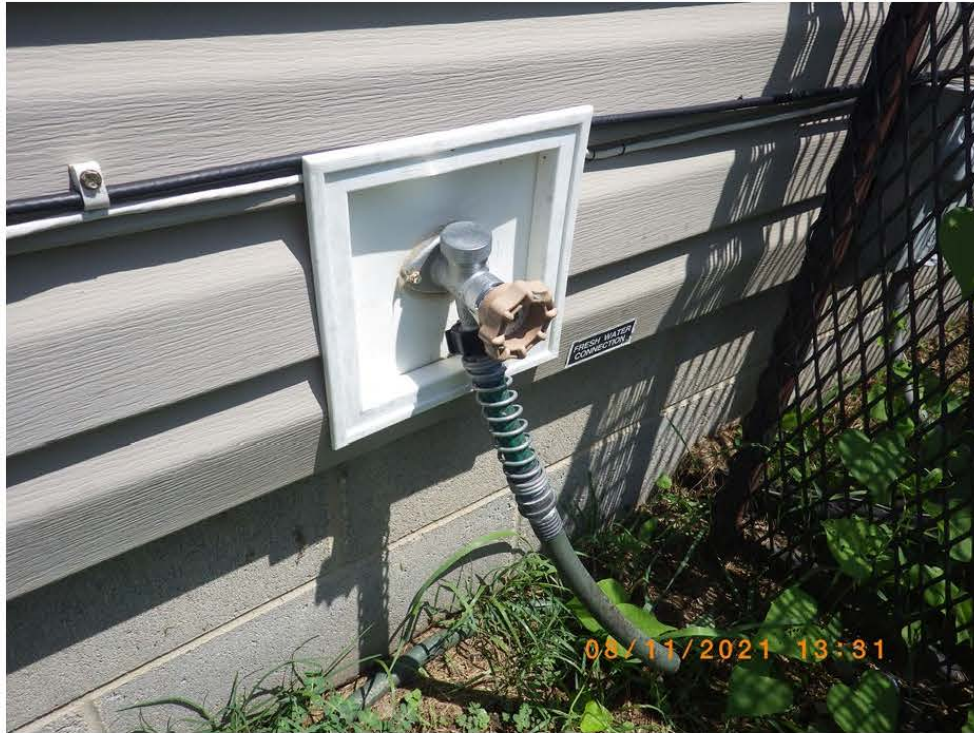
RIMG1470 Hose bib at site 1-08, 5620 Russell Ave, 8/11/21
