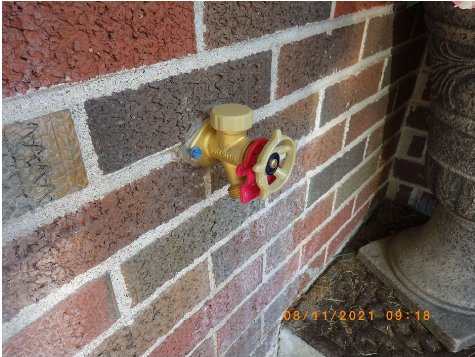
RIMG1463 Hose bib at site 1-01, 253 N 62 nd St. 8/11/21
