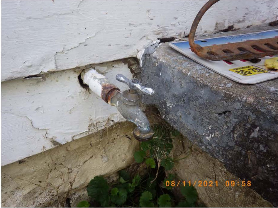
RIMG1464 Hose bib at site 1-03, 305 N 62 nd St. 8/11/21
