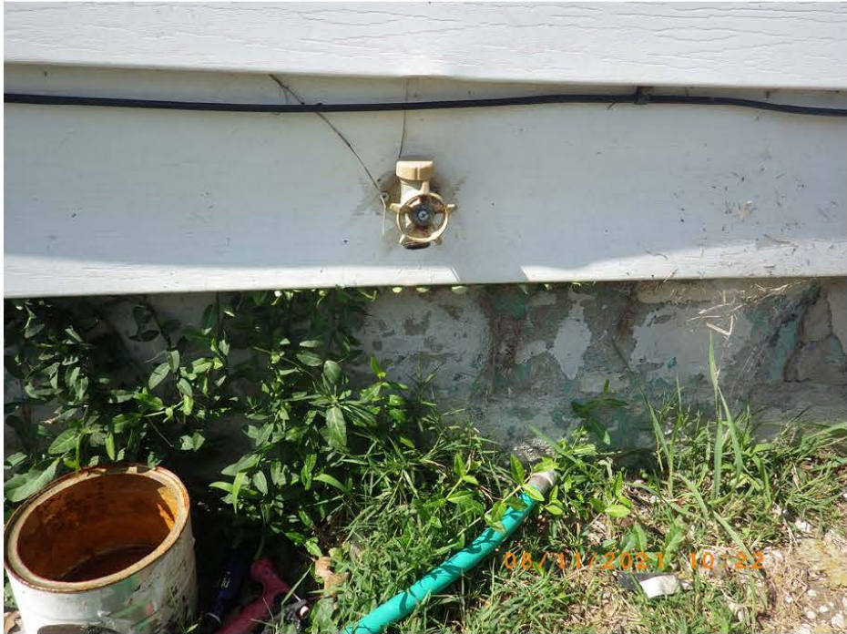
RIMG1465 Hose bib at site 1-04, 307 N 62 nd St. 8/11/21
