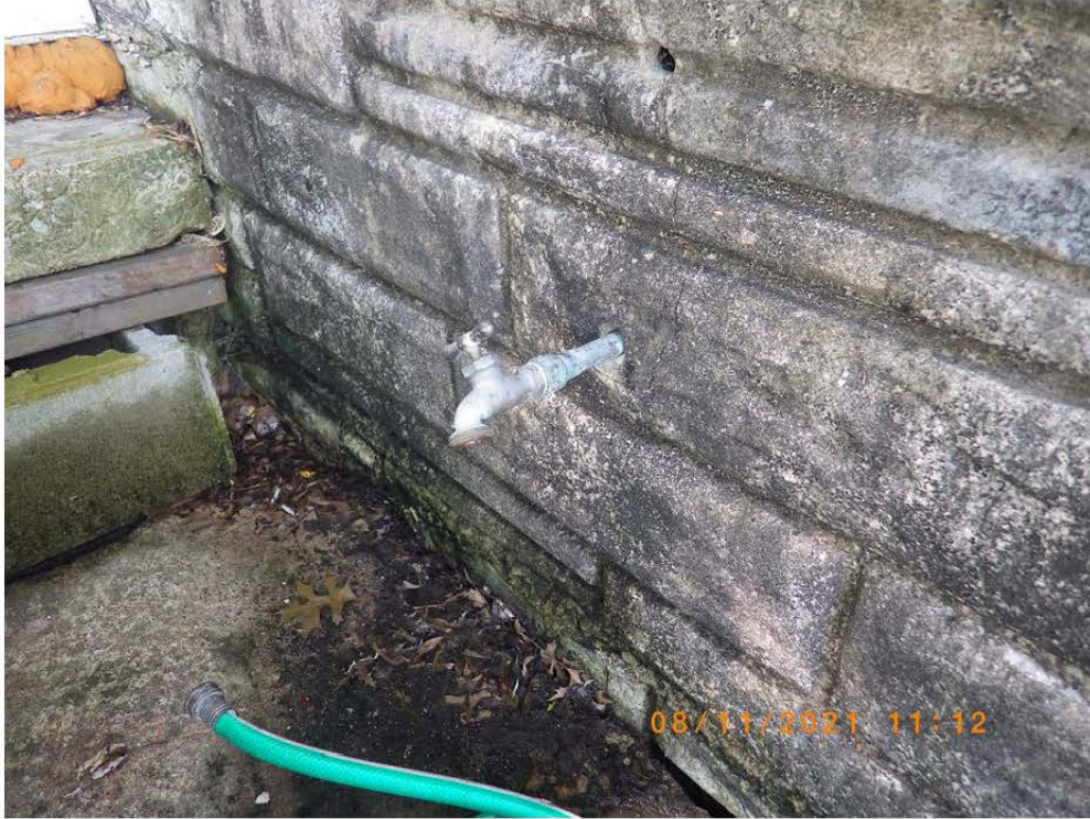
RIMG1468 Hose bib at site 1-06, 5951 Piat Pl, 8/11/21
