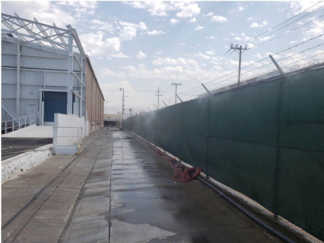
Perimeter Fence Misting System (6/17/21)
