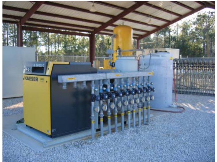
Air sparging system for groundwater treatment
