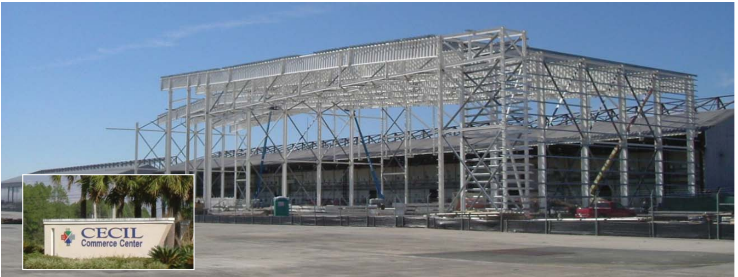
Construction of new hangar at the former Cecil Field NAS facility Inset: New sign at Cecil Commerce Center
