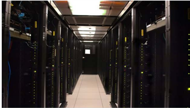
Figure 1. NREL's data center hot aisle containment system. Photo by Dennis Schroeder, NREL/PIX 18781.
