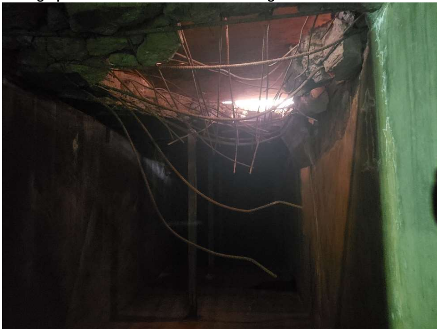
Photograph 1: South Tunnel Structural Damage
