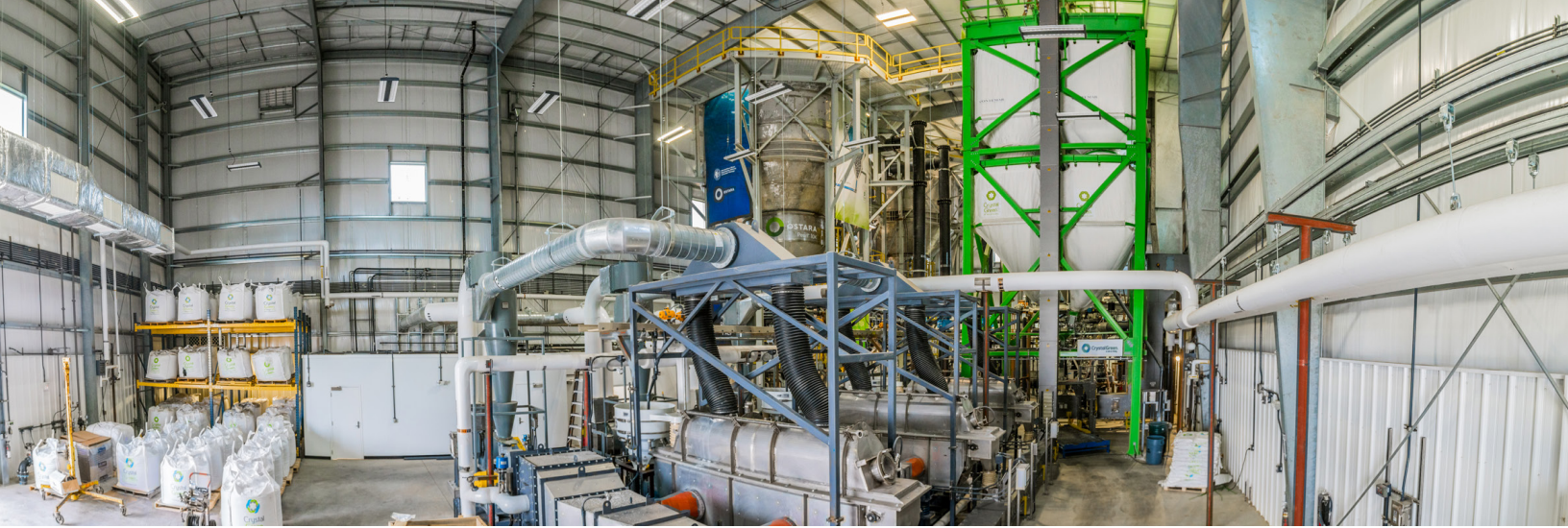
2017 Illinois PISCES Project: Metropolitan Water Reclamation District of Greater Chicago Phosphorus Recovery Facility
