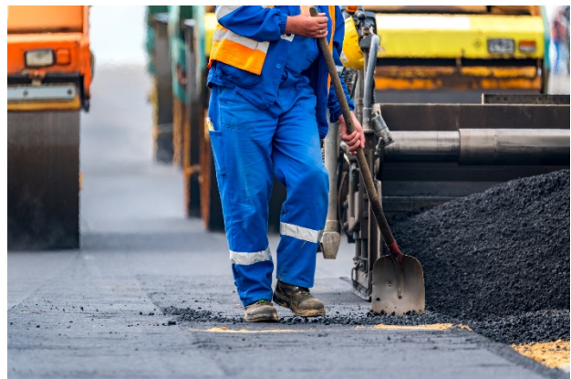
Routine maintenance, such as filling in potholes, repainting lane and edge lines, removing accumulated debris from drainage inlets, and mowing.
