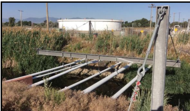
75,000 Barrel Floating Roof Tank & Feed Lines
