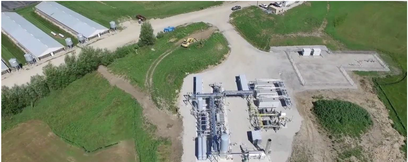
Biogas is transported through underground piping to a processing facility that removes impurities. Photo credit: Roeslein Alternative Energy, LLC
