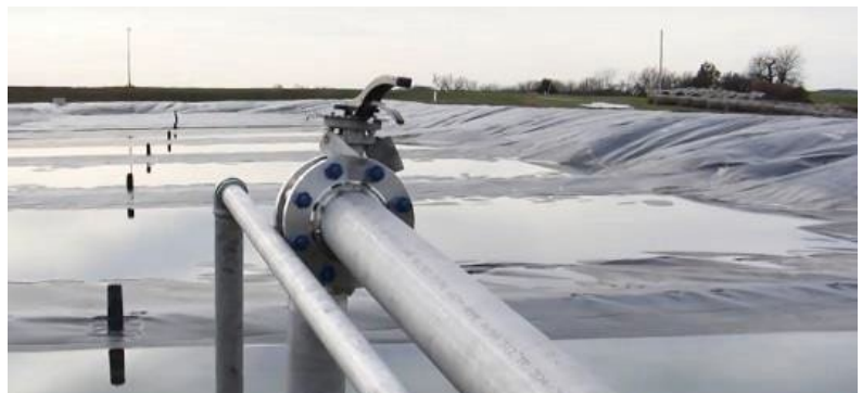
Biogas collection. Photo Credit: Roeslein Alternative Energy, LLC
