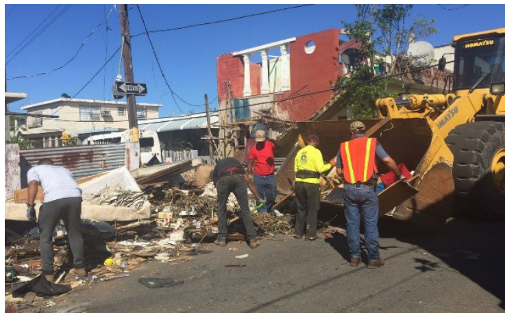
Street crews clearing debris in Puerto Rico after Hurricane Maria.
