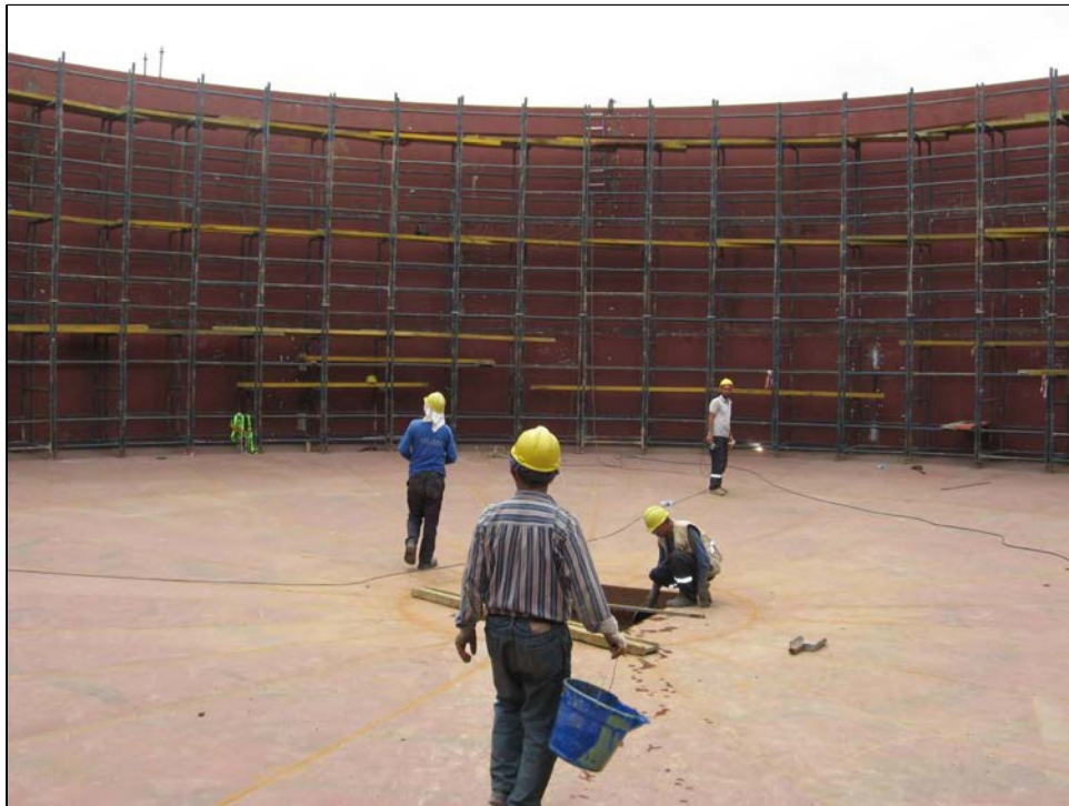
Photograph 2.2-8 Welded steel tank bottom with additional shell courses (interior).
