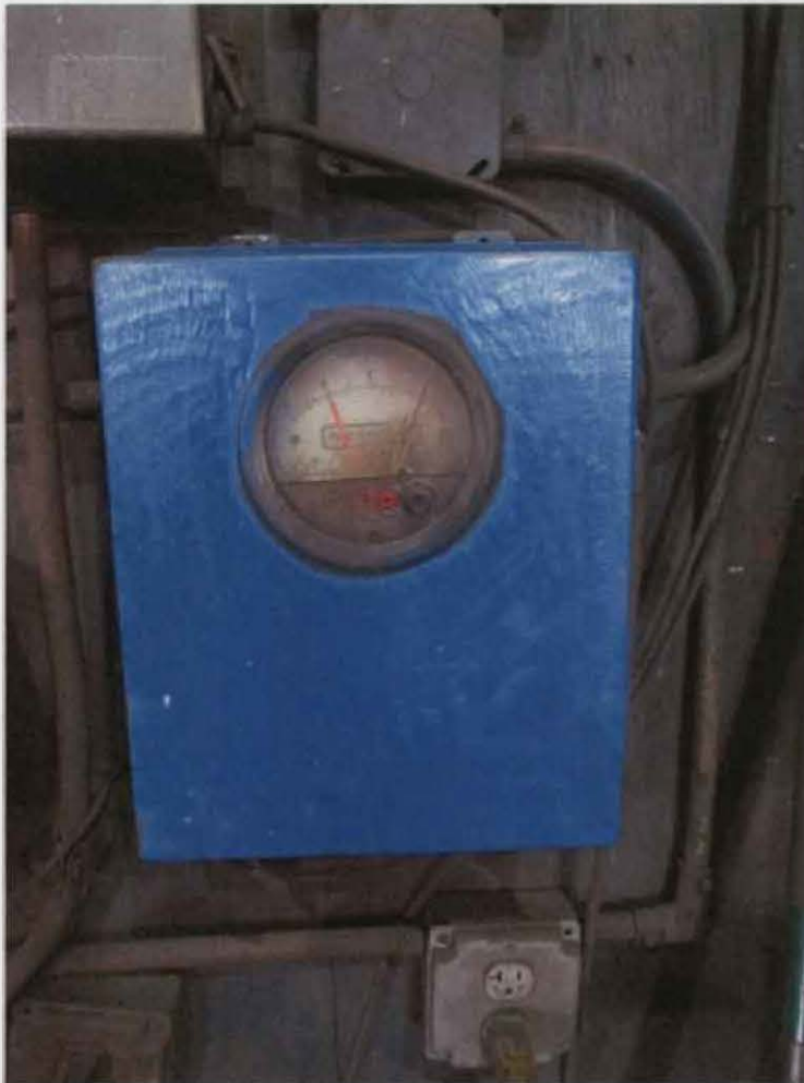
Photo 1. IMG_0359 at 8:10 am: The pressure drop device used for the Super Sack loading operations.
