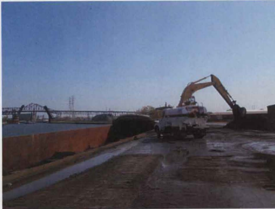
Photo 10. IMG_0370 at 9:01 am: SHB's water truck continually waters into the barge during DRI unloading.
