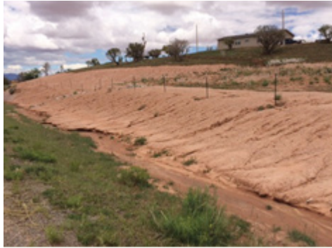
Before: Eroded soil at the base of the slope
