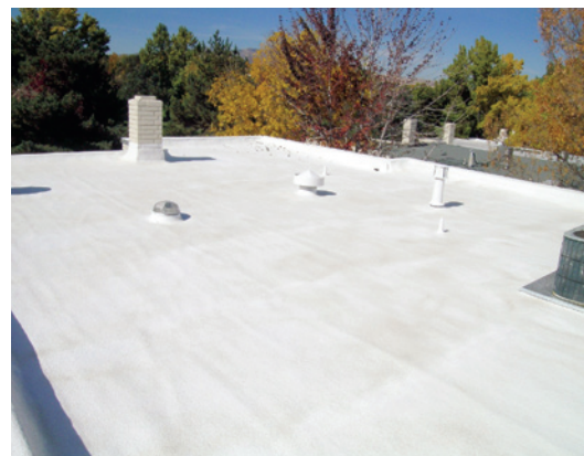
Figure 12: Cool Roof on a Condominium
