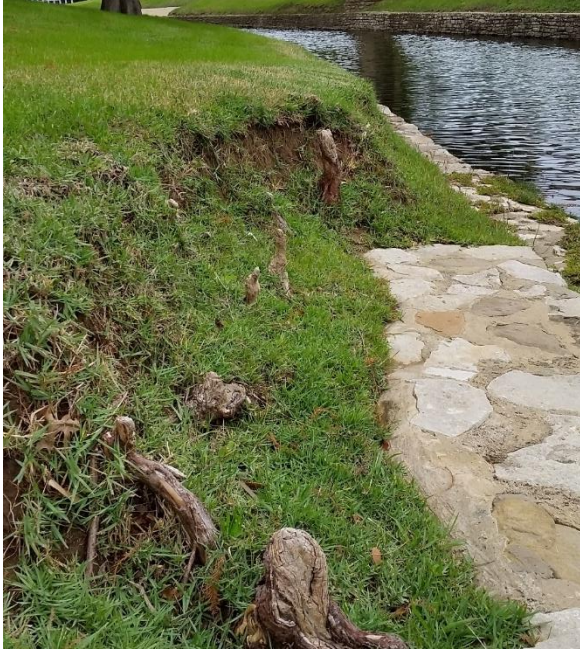
Figure 2 Erosion visible at water's edge
