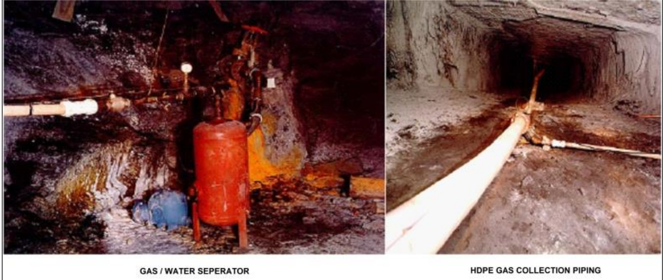
Exhibit 4-7: Gas Handling and Collection System
