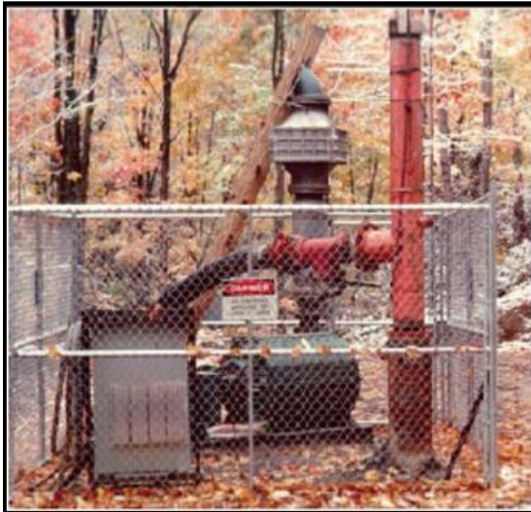
Exhibit 4-8: Vacuum Pump - Vertical Gas Gob Well
