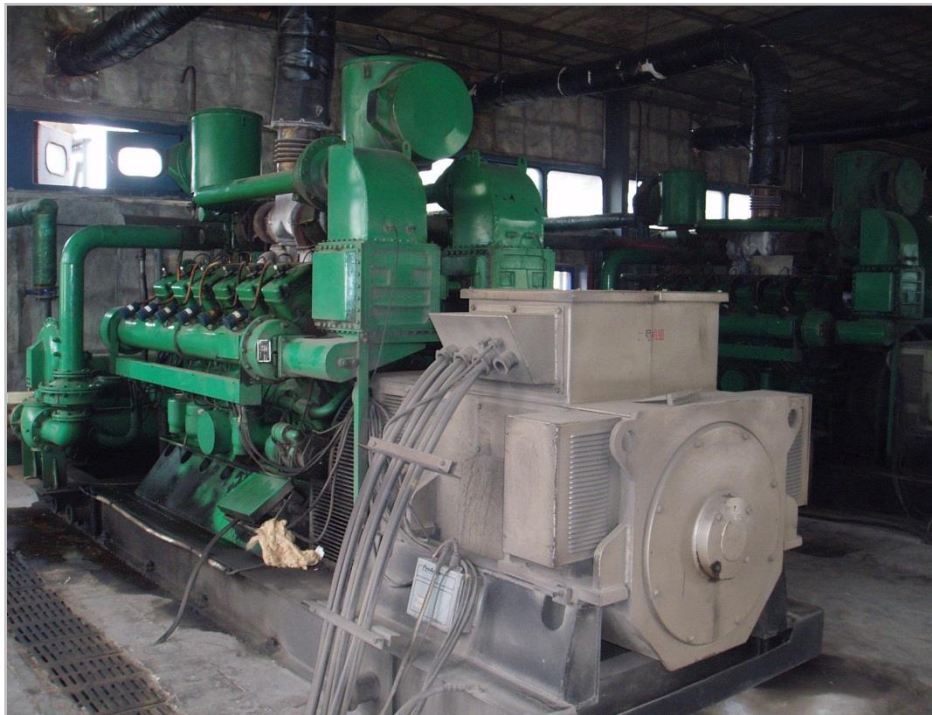
Exhibit 5-3: 500 kW Shengli Oil Company CMM Generator Set
