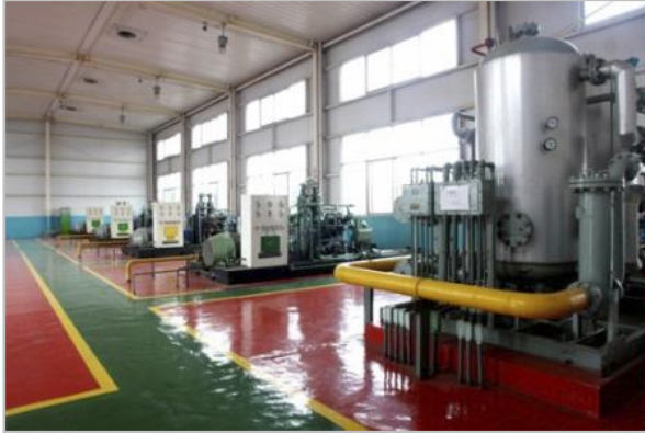
Exhibit 5-10: CNG Compressor Station
