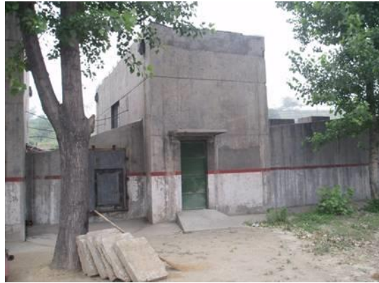
Exhibit 1-18: Main Surface Fan Infrastructure at Mine No. 6.
