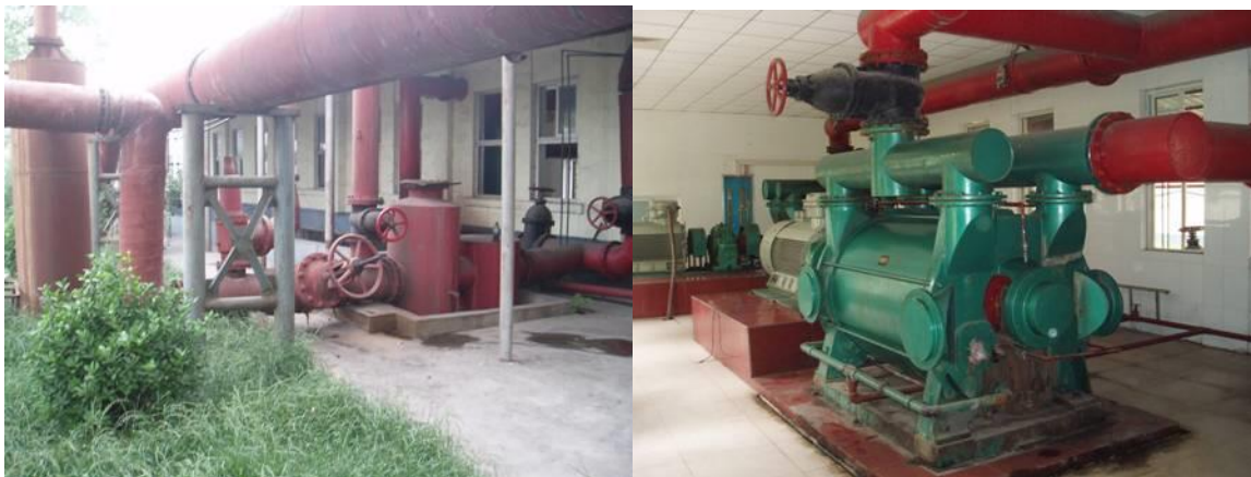
Exhibit 1-9: Surface Gas Collection and Water Separation (on left), Vacuum Pump (on right)
