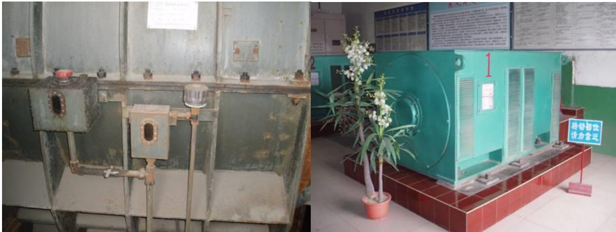
Exhibit 1-19: Fan Housing with Sensors (left) and Electric Motor (right).
