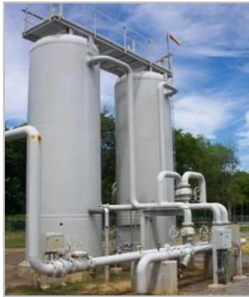
Exhibit 5-7 SulfaTreat Vessels (Pena, 2007)
