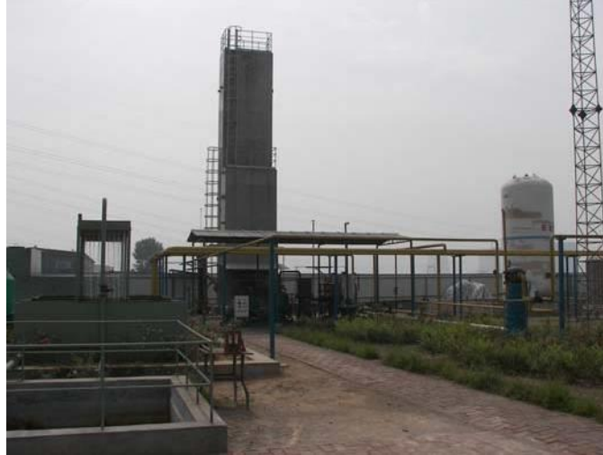
Exhibit 5-15: Yangquan CMM pilot project - refrigeration tower (left) and LNG storage tank (right) (Yang, 2008)
