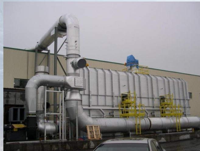
Asphalt Shingles - COC emissions Joliette, Quebec, USA 35,000 cfm
