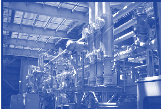
After: ITC Holdings Corp. replaced the leaking GIS at the St. Antoine Substation with new equipment supplied by Mitsubishi Electric.
