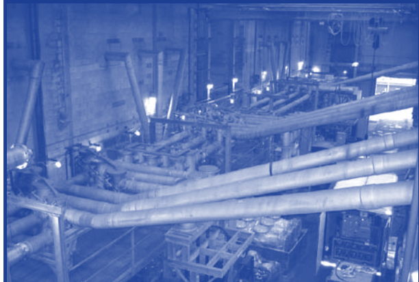
Before: Leaking GIS at the St. Antoine Substation.
