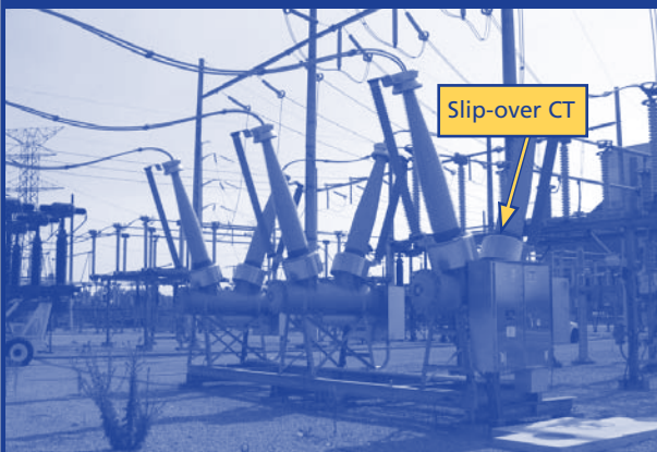
After: Replacement 300-SFMT-63E Gas Circuit Breaker with fewer fittings and a simpler design. The newer style gas breakers utilize slip-over CTs on the outside of the bushings that do not require gas insulation.
