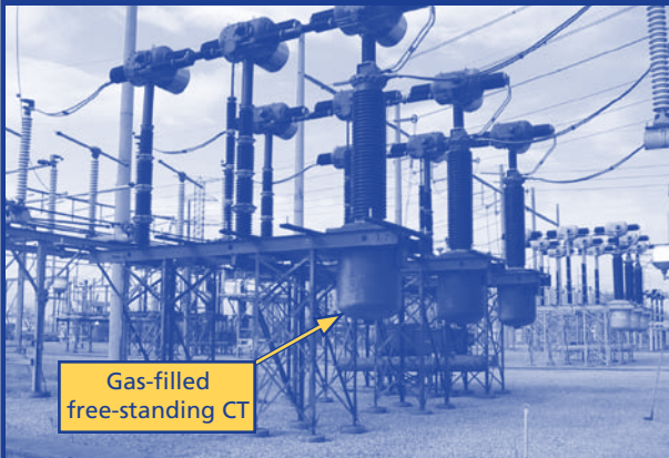
Before: Leaking GE ATB-7 Circuit Breaker that uses a separate gas insulated current transformer (CT).
