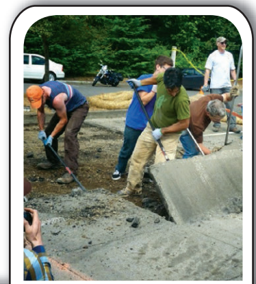
Volunteers remove pavement to make way for a new Parking Forest. See article on page 12 .
