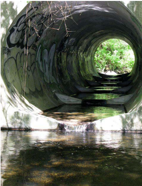
Before this culvert in Santa Cruz County was retrofitted with concrete baffles, water shot through its smooth barrel at high speed, making it very difficult for fish to swim upstream. (Photo by Eileen Ecklund)
