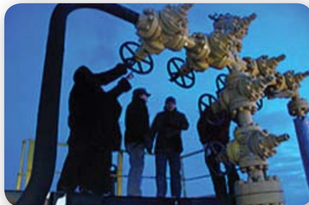
Gas valves at Russia's Yamburg gas production and processing site.
