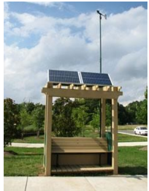
South Regional Library Pilot Station in Durham, NC
