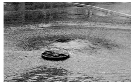
SSOs can occur at numerous locations in the sewer system, including at manholes.
