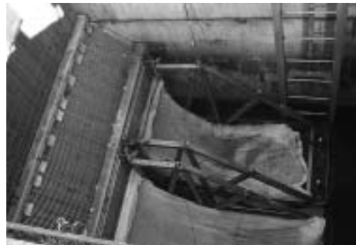
Photo: Solids and floatables controls, such as the nets pictured here, are installed at all North Bergen CSOs. Courtesy of NJDEP
