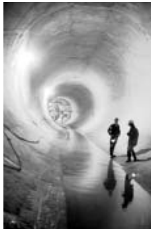
Photo: New deep rock tunnel, part of Chicago's extensive Tunnel and Reservoir Plan (TARP). Courtesy of MWRDGC
