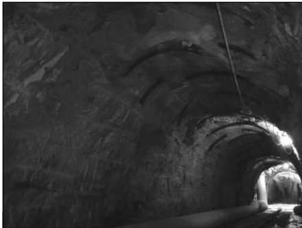
CSO controls can be costly to implement. Construction of the 7.2 mgd storage tunnel in Richmond, VA cost more than $29 million. The tunnel is one component of a three-phased program.
