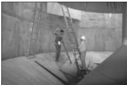
Planning and budgeting for operations and maintenance procedures is needed to ensure that expensive capital equipment, such as this vortex separation system in Columbus, GA continues to function properly.
