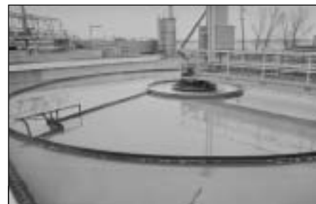
Like most cities, Chicago maintains excess primary treatment capacity to accommodate wet weather flows. Shown is a primary clarifier at a Chicago-area POTW.
