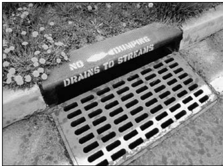
Storm drain stencil project in a New Jersey CSO community. Most CSO permittees generally follow the concept of the NMC in their CSO control programs.
