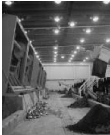
Photo: Trash screens at Atlanta's Intrinishment Creek CSO Center. Courtesy of Atlanta Department of Public Works
