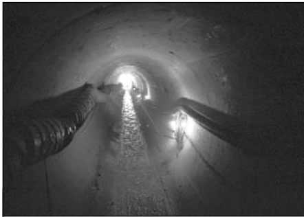
Sewer separation tunnel installed by New Brunswick, NJ. Sewer separation is the most common long-term control used by CSO permittees.
