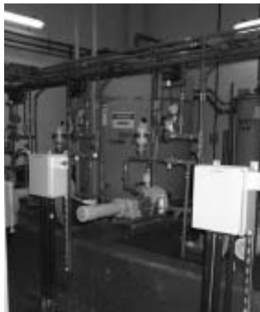
Photo: New dechlorination system at the Cottage Farm POTW. Courtesy of MWRA.
