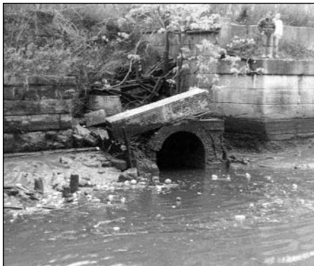
Addressing deteriorating infrastructure, such as this crumbling CSO outfall, is one aspect of most CSO control programs.
