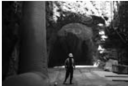
Photo: Construction of a 6.7 million gallon storage tunnel along the Falls of the James. Courtesy of Richmond DPU
