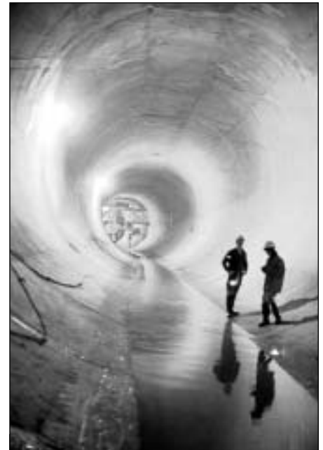
Chicago had one of the nation's earliest large-scale CSO control programs. As of 2001, Chicago's Tunnel and Reservoir Project (TARP) has cumulatively captured 565 billion gallons of combined sewage that would otherwise have flowed to area receiving waters.
