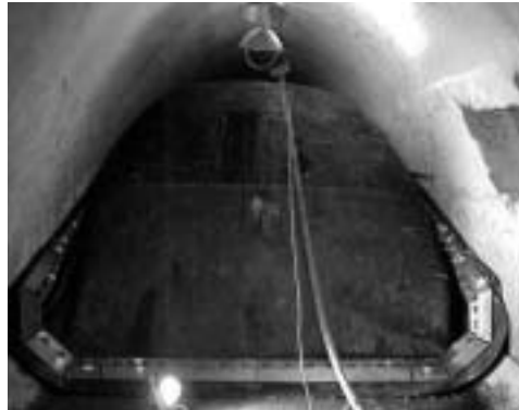
Photo: Inflatable dam at the Sneads Branch CSO. Courtesy of LJCMDS
