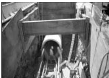
A new line is installed as part of a sewer system separation project in New Brunswick, New Jersey.
