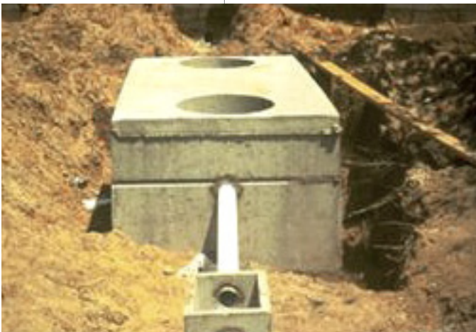
Septic tank and distribution box
