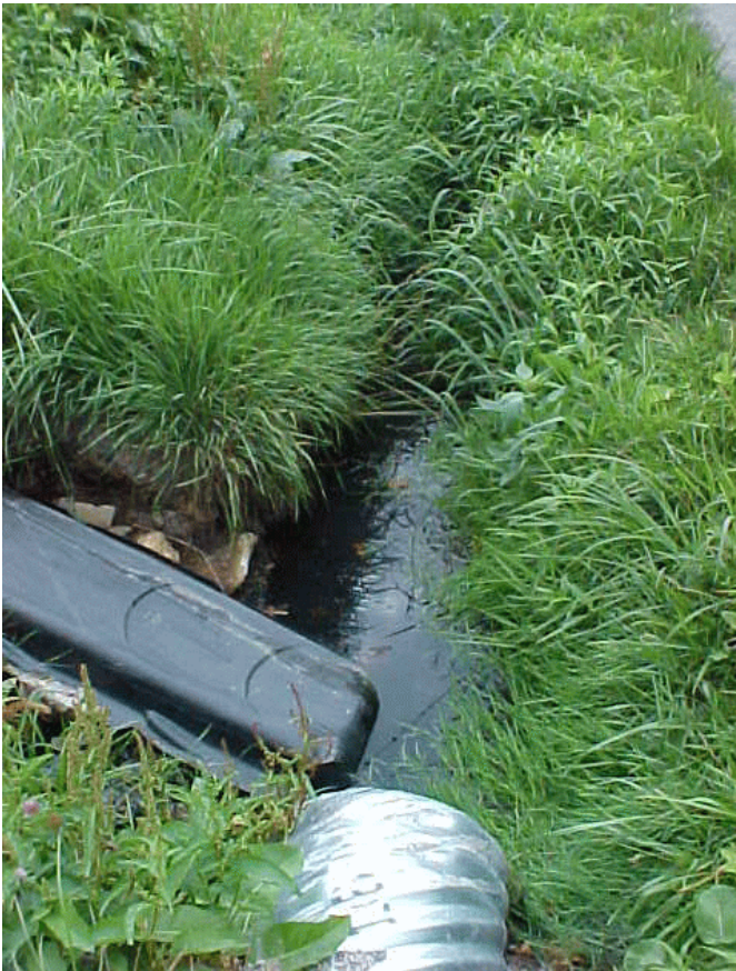
Straight Pipe Drainage: Path Fork, Kentucky (Harlan County)
