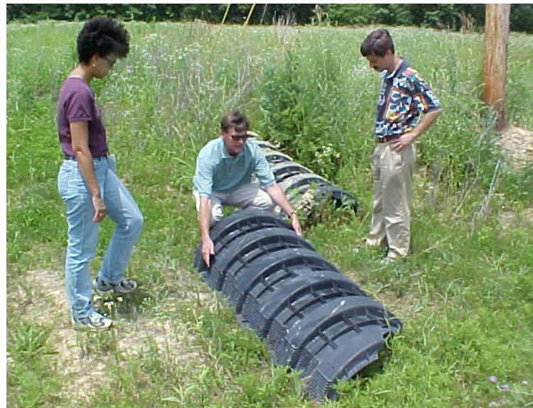
Infiltrator Drainage System: Preston, KY
