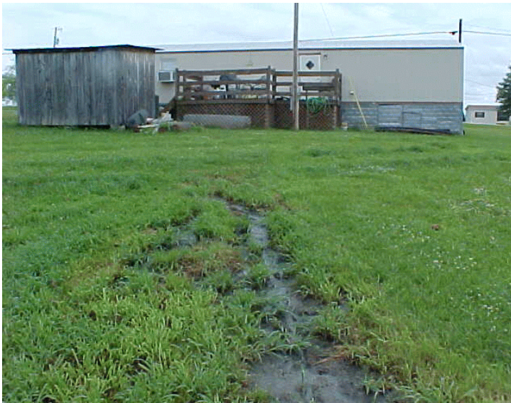
Failed Septic System: Preston, KY
