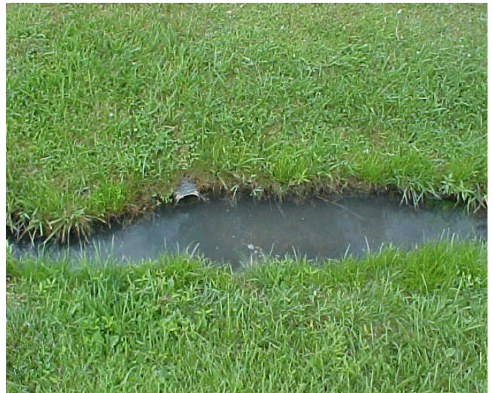
Septic drainage: Preston, KY
