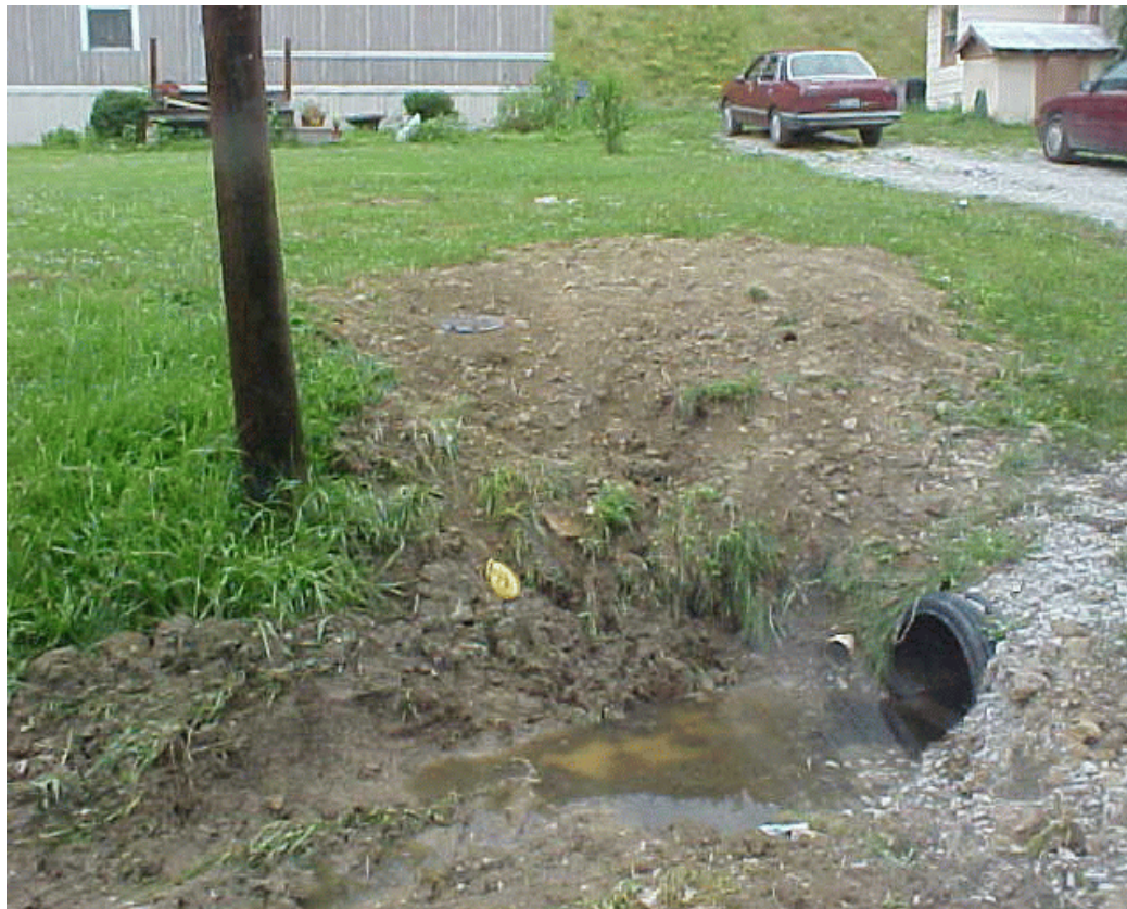
Straight Pipe:Martin County, KY
