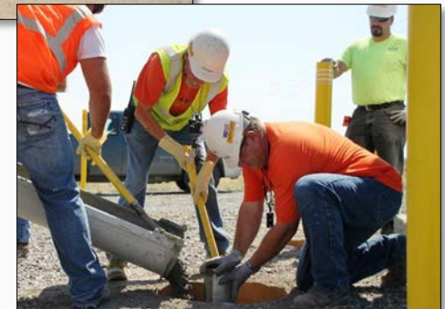
Groundwater extraction well
